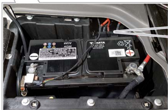
Battery under driver's footwell
